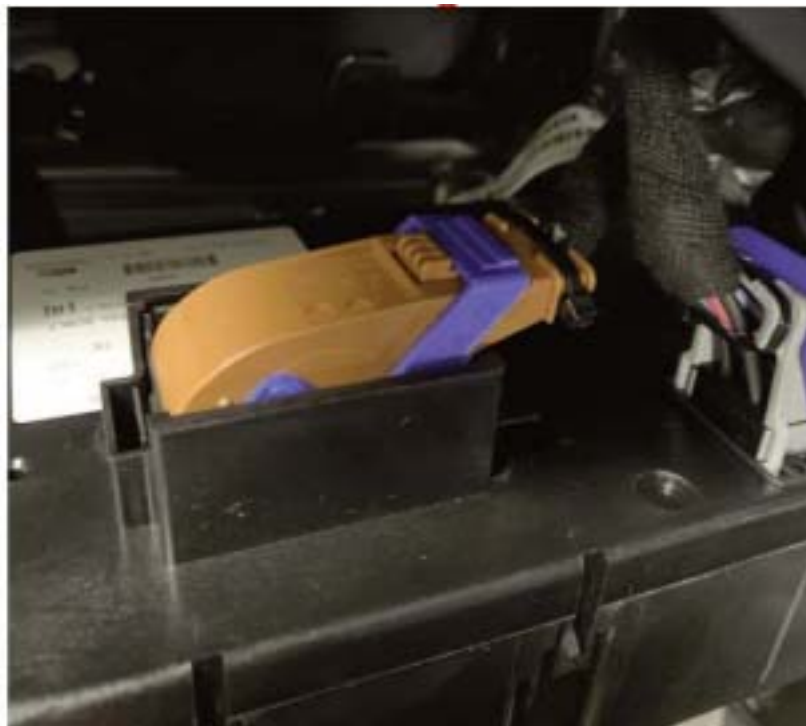
BCM Brown connector in rear of BCM/fuse box 60 pin plug. Rostra Red ignition wire connect to DK. Blue wire in position 12.
